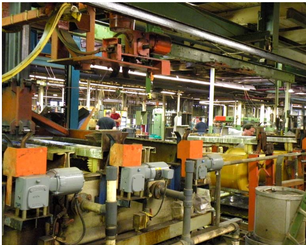
Still going strong. This computer-controlled automatic barrel line was installed in 1997.
